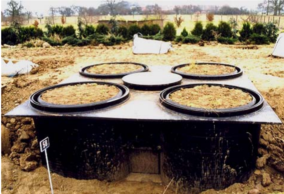
Figure 3. Polyethylene (PE-HD) lysimeter station with four lysimeters in a clover leaf arrangement with an entering hatch (center position) during the installation process.
